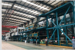
• 彩涂卷生产线 PPGI COIL PRODUCTION LINE
